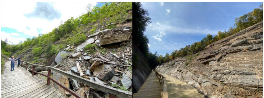
Figure 16, Paw Paw Slope Stabilization Project – As viewed looking south at the 2016 rockslide (May 2021 on left and October 2023 on right)
