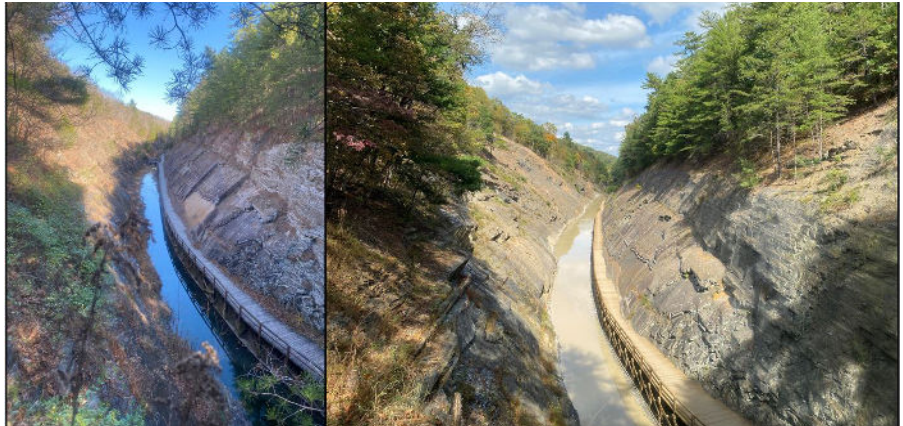
Figure 14, Paw Paw Slope Stabilization Project—As viewed from above the north portal of Paw Paw Tunnel (November 2020 on left and October 2023 on right)
