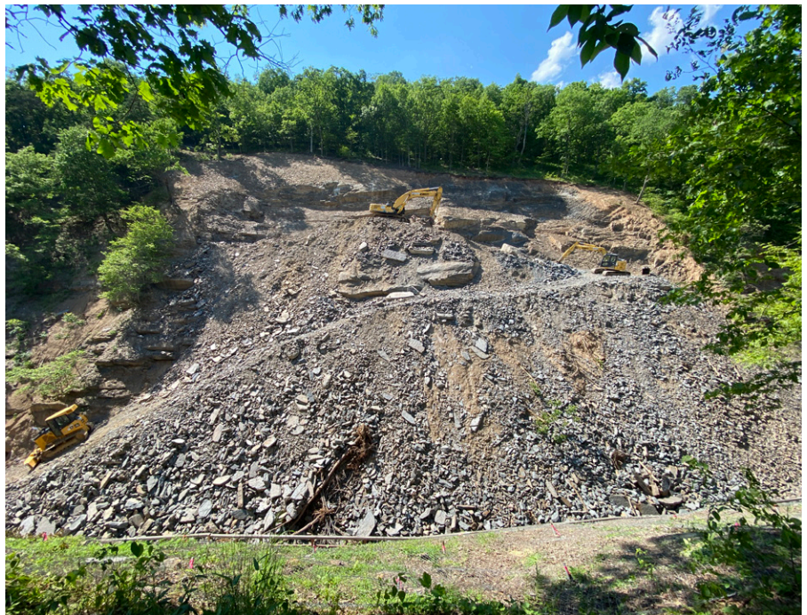
Figure 11, Establishment of switchbacks and removal of additional slope concern area and 2016 rockslide
