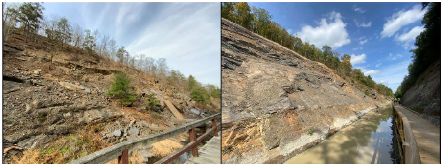
Figure 15, Paw Paw Slope Stabilization Project – As viewed looking north at the 2016 rockslide (November 2020 on left and October 2023 on right)
